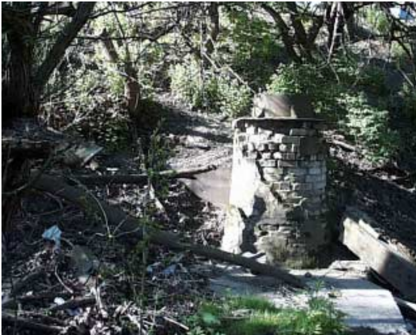
Figure 5.2.3: Manhole in NMR with Structural Deficiencies
