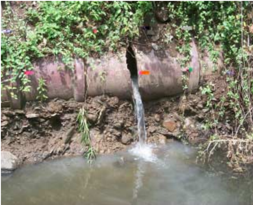
Figure 5.2.2: Cracked Pipe in the NMR Sewer System
