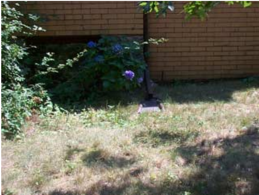
Figure 4.3.10: Disconnected Downspout with Splash Block
