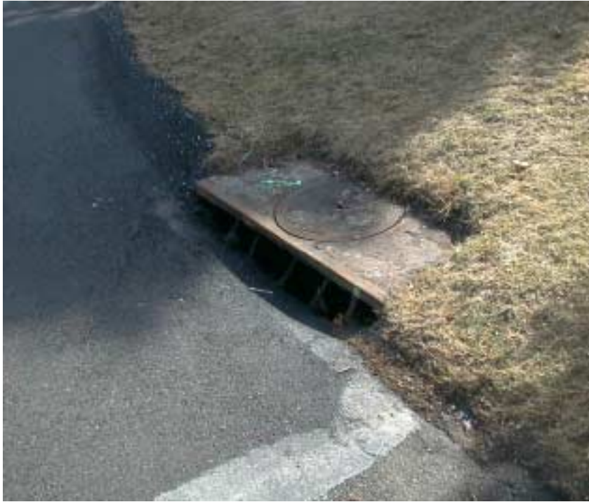
Figure 4.3.5 Typical Catch Basin in NMR
