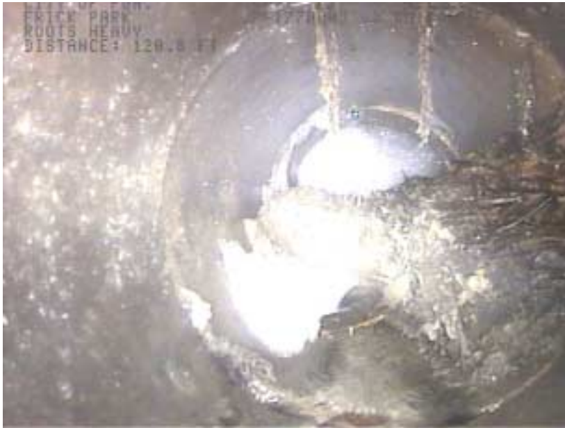
Figure 4.3.6: Root Intrusion in NMR Trunk Sewer
